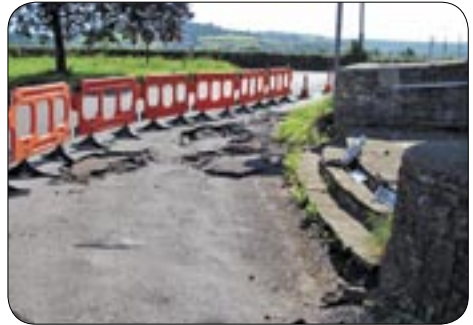
Repairs to the county's roads will cost over £25m
